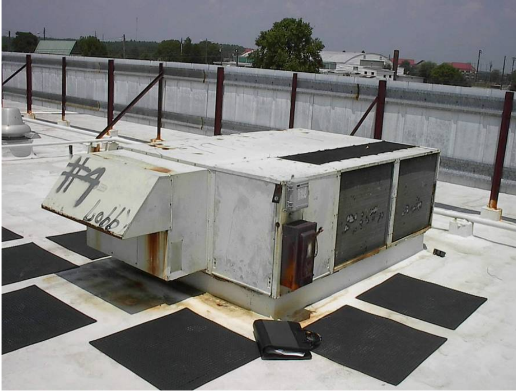
Figure 3. Fort Gordon RTU Replaced as Part of Demonstration
