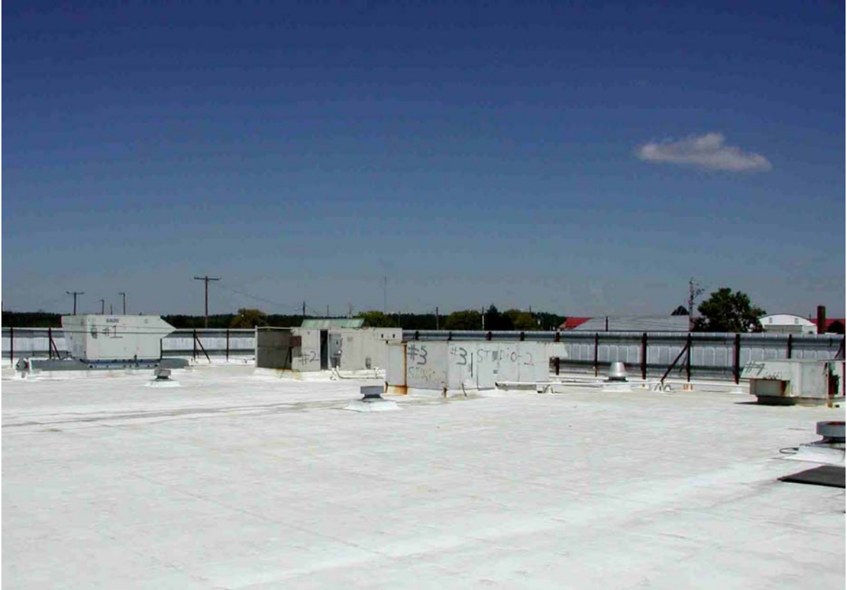
Figure 2. Rooftop View from the South of the Fort Gordon Club's North Wing.
