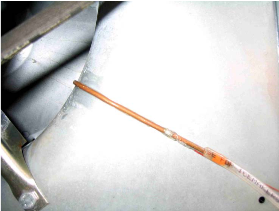
Figure F-6. View of supply fan inlet bell showing the throat pressure tap.
