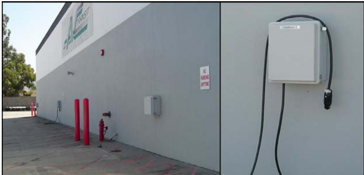
Figure C-7. Fuel cell bus/battery charging station at AC Transit
