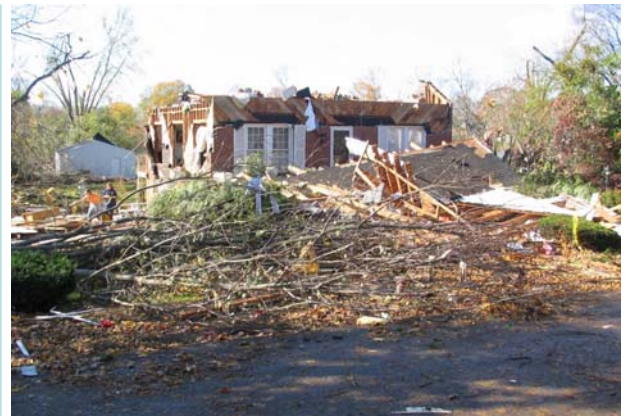
F2 tornado damage in Munfordville, KY, November 6, 2005
