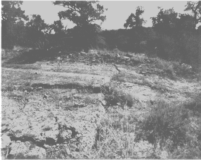
Figure 4. Photograph of surface crack through bedrock.
