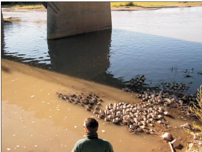
Figure 2. (A) Single A-Jack (Photograph by T.A. Kenney), (B) A-Jacks module installed at Green River Bridge at State Road 19 (Photograph by T.L. Ularich), and (C) a portion of the A-Jacks matrix at Green River Bridge at State Road 19 during low flow conditions, October 2003 (Photograph by T.L. Ularich).
