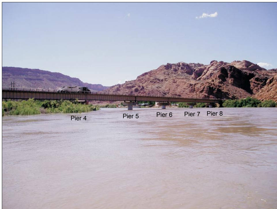
Figure 7. Downstream view of the Colorado River Bridge at State Road 191, 2005. (Photograph by T.A. Kenney)
