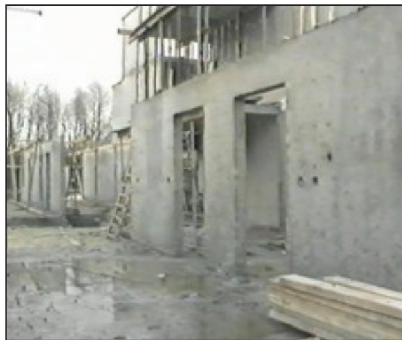
All walls appeared to be perfectly smooth after removal of the shuttering elements.
