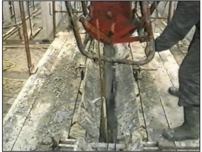
A number of walls were poured in both blocks of houses using a concrete bucket.
