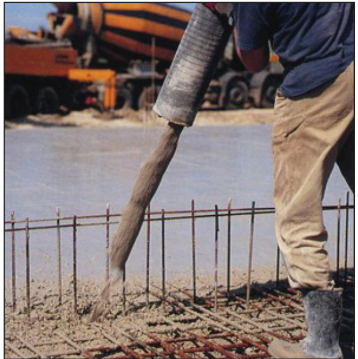
In order to demonstrate the workability of Aardelite's round shaped gravel during pumping, one concrete pour was executed with a concrete pump.
