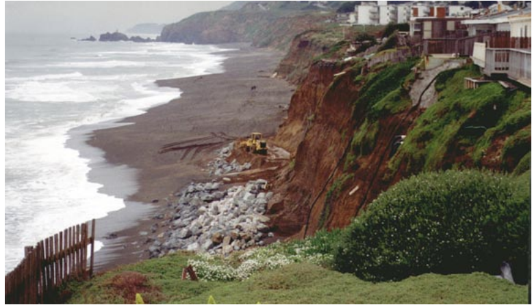
Photograph taken just before the 1997-98 El Niño storms, looking northward along the approximately 30-m-tall seacliff at North Esplanade Beach in Pacifica, CA. The soft cliff shows signs of erosion, and a rip-rap seawall is being constructed at the cliff base to protect houses along the cliff edge. The seawall was not completed before the storms, and the cliff retreated more than 10 m. Most of the houses along the cliff were condemned and razed after the storm season.
