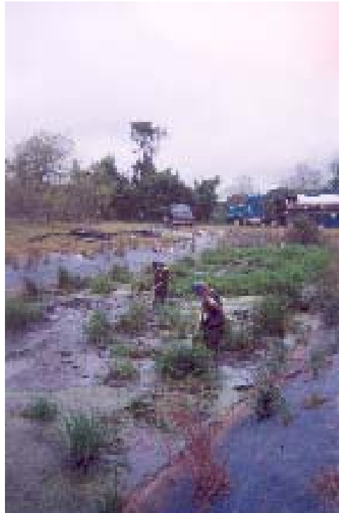
Figure 1: Pumping of Surface Water
