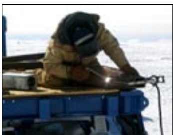
Welder Edgar Vega makes a visit from McMurdo Station to Taylor Dome to help repair ITASE equipment before the traverse began.
