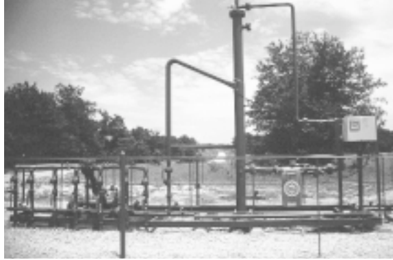
Surface equipment for 2-phase separation (gas and liquid) that is operated in Southern Oklahoma by Chevron. DOE is currently experimenting with a 3-phase separator.
