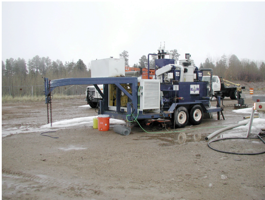
Fig. 9. The Los Alamos mud cleaning system includes a shale shaker, settling tank, and hydrocyclone mud cleaners. The cleaner was manufactured by TriFlo to meet the needs of the trenchless utilities industry. It has been upgraded by Los Alamos to improve the performance of the cleaning unit to reduce mud-pump wear.
