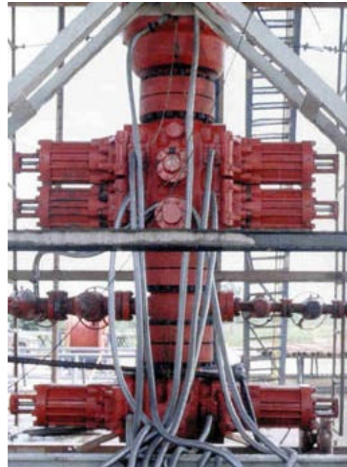
Fig. 1. Blowout preventer stack (BOP)
