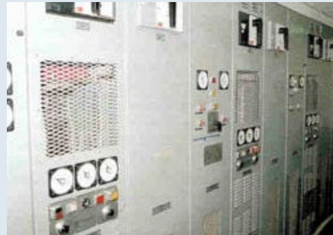
Fig. 7. Electric control panel
