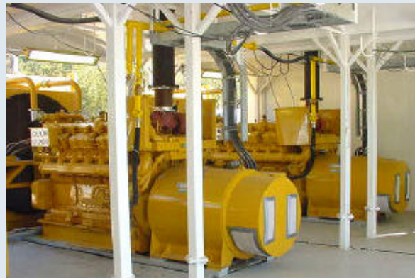
Fig. 10. Engines and generators
