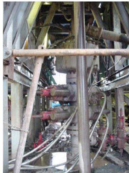
Fig. 1. Blowout preventer stack
