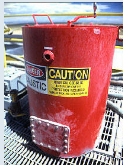
Fig. 6. Caustic soda mixing container
