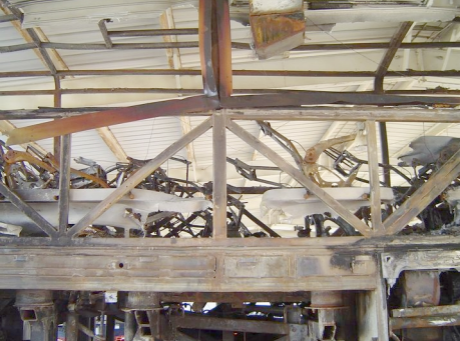
Fire Photo #15 - Missing Section of Right Side Return
