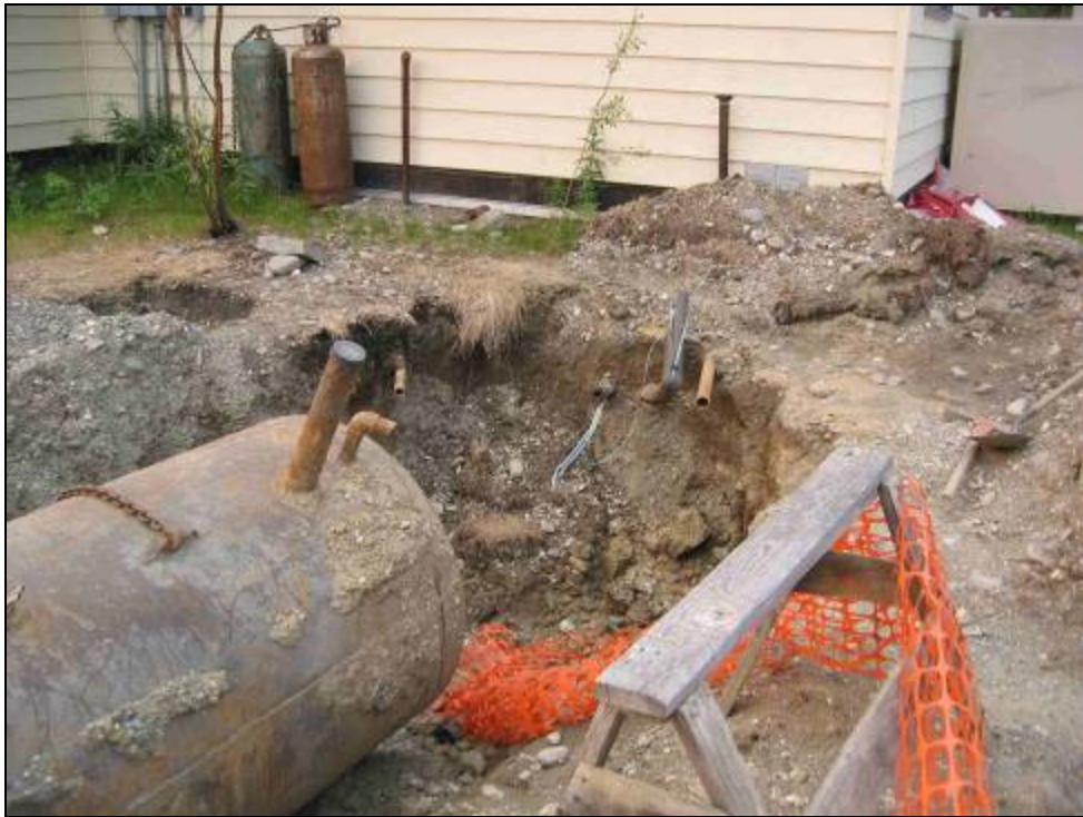
A tale of two spills: absorbent pads are deployed to soak up fuel from overflowing the underground fuel tank (top), while chronic leakage from faulty original installation was discovered when excavating the tank....nevertheless, it's a pretty functional bunkhouse!!! (photos by C. Knight (top) and B. Raften)
