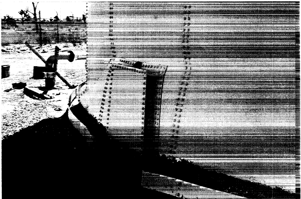
Figure 9.7 CSA-70 clean-out door, tank on rock foundation.
