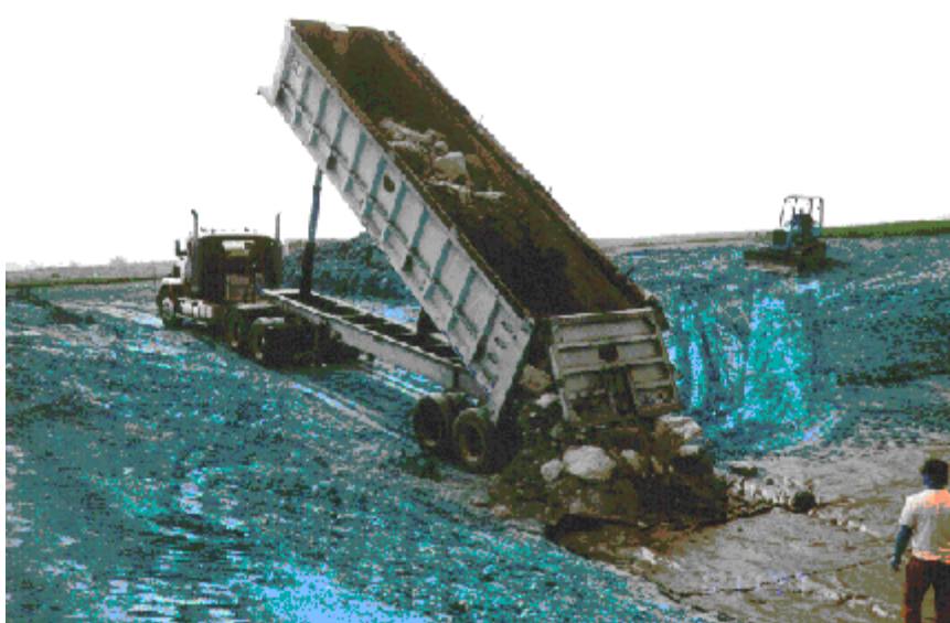
Figure 9. Truck Unloading FGD.
