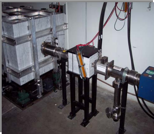
Figure 1. Collimator C836B, bellows, marble mask, Loss Monitor LM8C1 beside 836 marble mask with loss monitor LM8C3 above on wall, position monitor HP837, gradient magnet.
