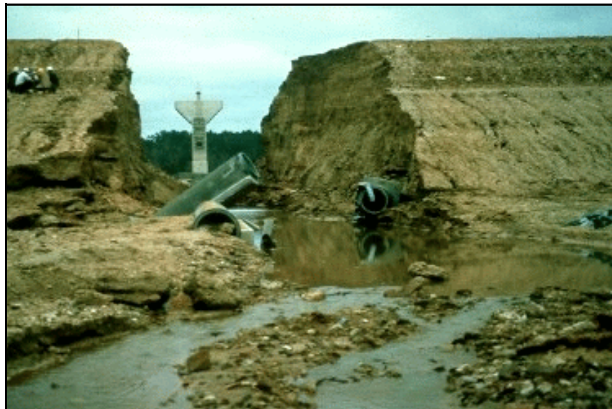
Figure 85. —This embankment dam constructed with dispersive clays failed on first filling of the dam.
