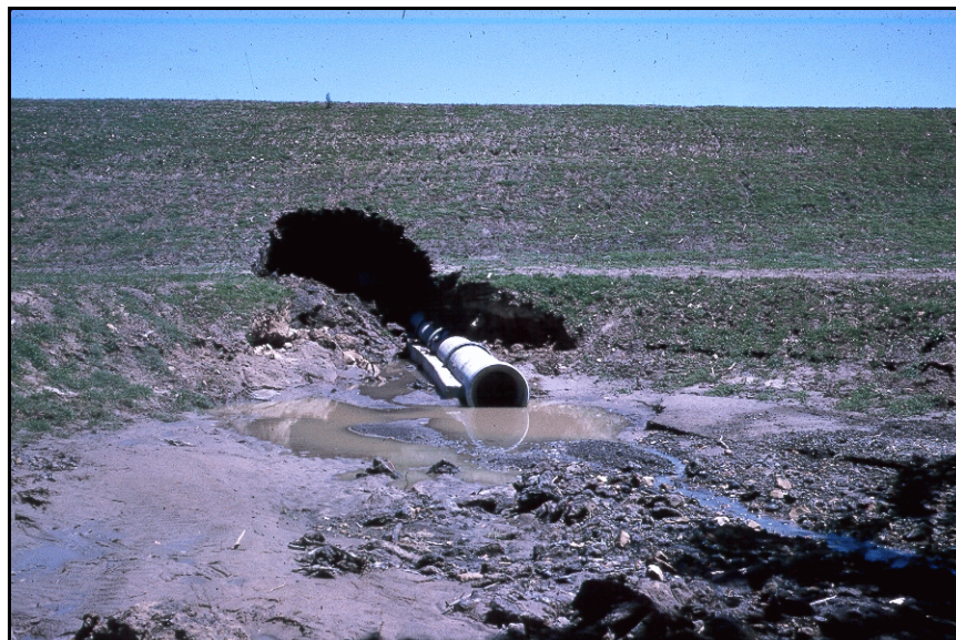
Figure 104. —Failure of an embankment dam due to internal erosion of hydraulic fracture cracks upon first filling of the reservoir.
