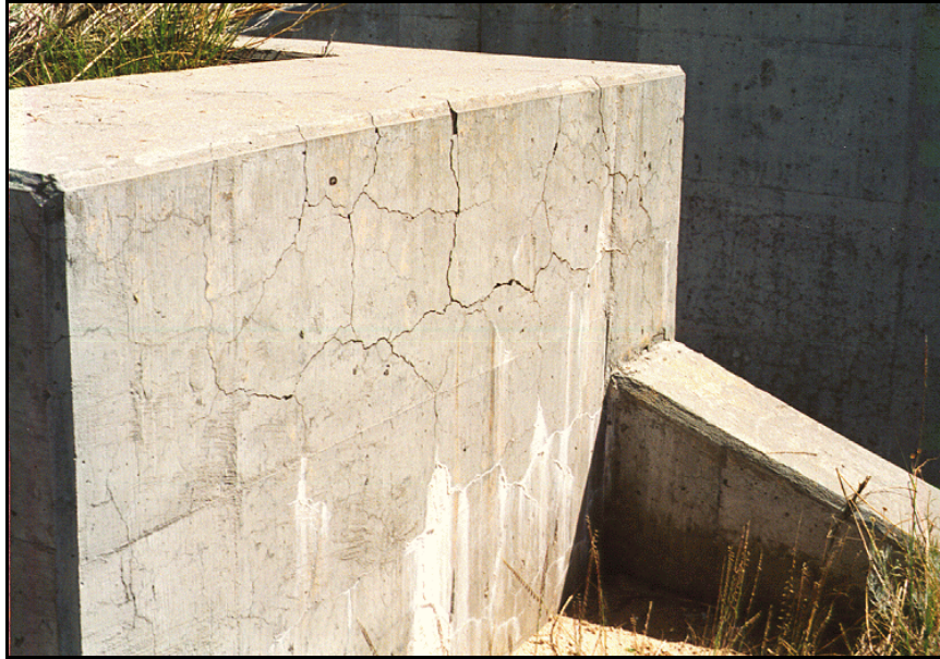
Figure 107. —Concrete deterioration from alkali-aggregate reaction.
