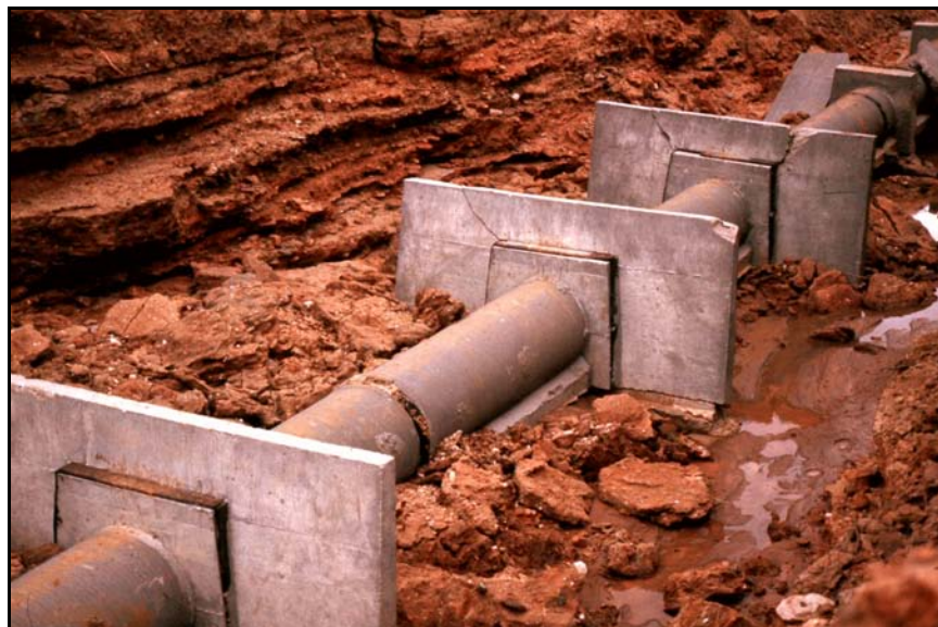
Figure 102. —Conduit with intact antiseepage collars. The collars would have interrupted flow along conduit. Internal erosion or backward piping erosion likely occurred through hydraulic fractures in surrounding earthfill, resulting in failure of this embankment dam.
