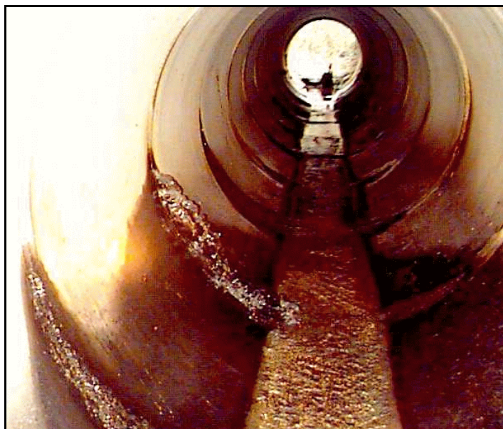
Figure 96. —Leaking joints in a 60-inch diameter RCP spillway. Several large voids were also observed in the adjacent earthfill on the upstream slope.
