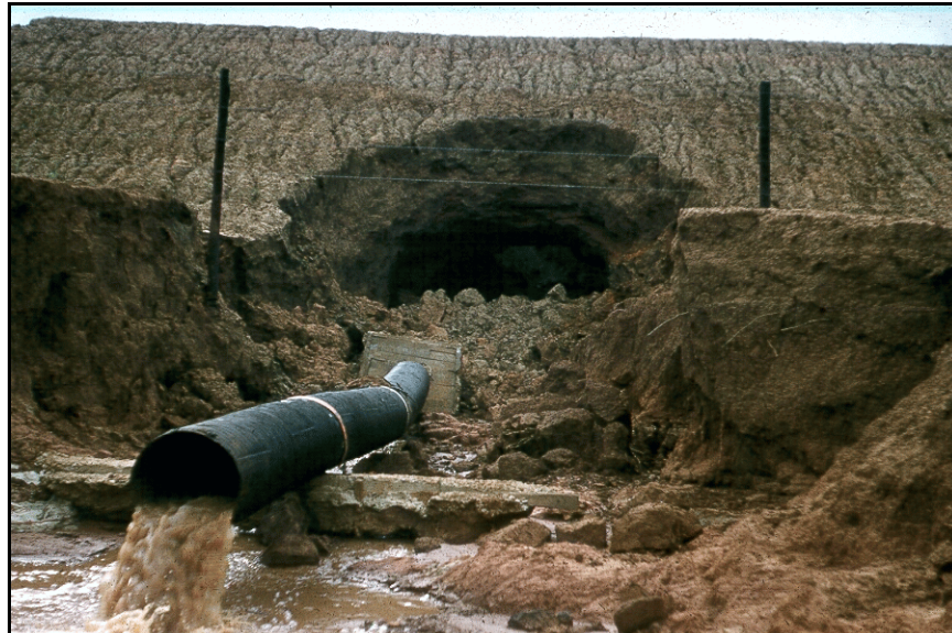
Figure 84. —An embankment dam in Mississippi constructed of dispersive clay soil, failed on first filling with low reservoir level. Failure was likely caused by cracks from differential settlement, hydraulic fracture, or poor compaction about the outlet works conduit. This embankment dam had no filter.
