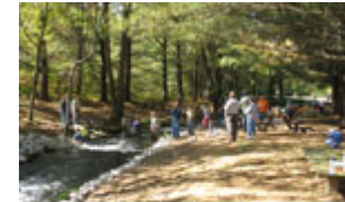
Conservation Project - Riprap placed along eroding streambanks of hatchery effluent canal. FWS photo.
