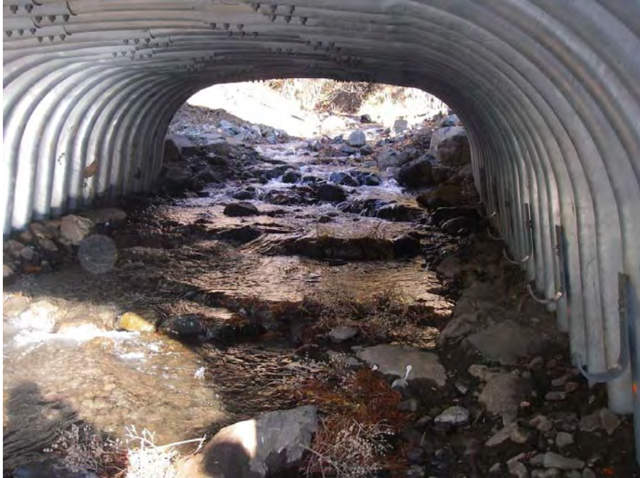
Photograph No. 11. Creek bed inside of the bottomless arch culvert. Photo by J. Chan, Reclamation.
