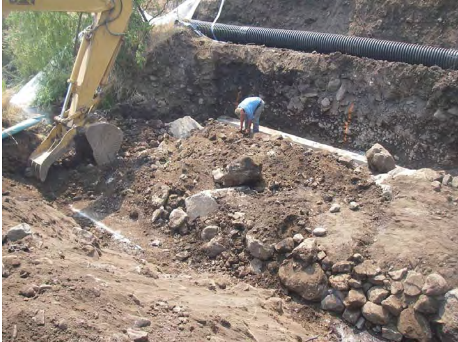
Photograph No. 7. Left side footers in place and completing installation. Photo by J. Farver.
