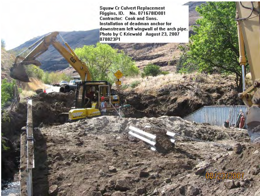
Photograph No. 8. Installation of deadman anchor for downstream left wingwall of arch pipe. Photo by C. Kriewald.
