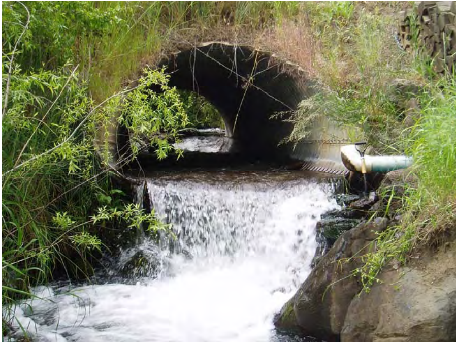
Photograph 1. Squaw Creek culvert downstream side north bank before project construction. Photo by: D. Weigel, Reclamation.
