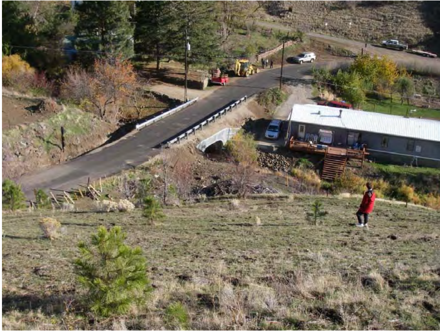
Photograph No. 13. Completion of the project site showing curbing and guardrails installed along the road bed, the bottomless arch culvert covered with road fill and the road re-paved with asphalt. Photo by J. Chan, Reclamation.
