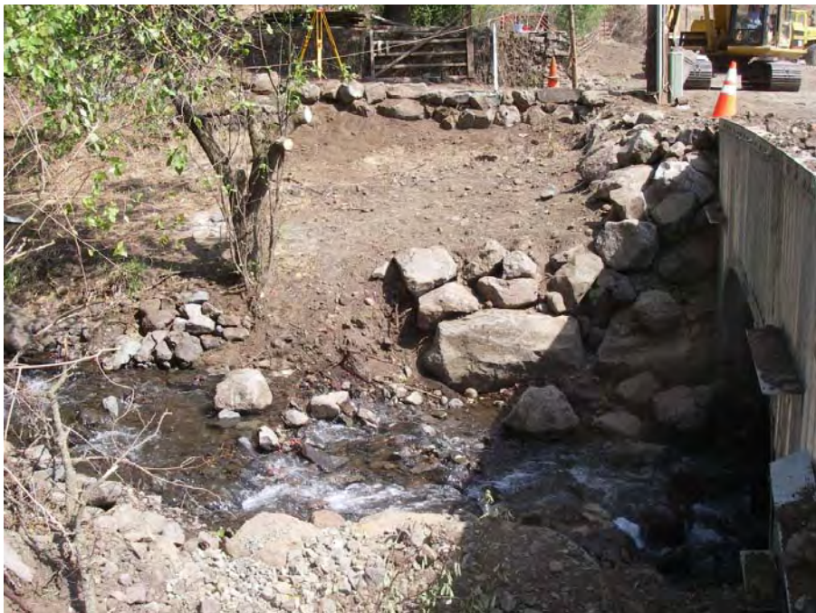
Photograph No. 12. Looking at the upstream side of the bottomless arch culvert showing retaining wall and riprap on creek bank. Property owner's driveway is accessed thru open gate at the top and center of photograph. Photo by J. Chan, Reclamation.
