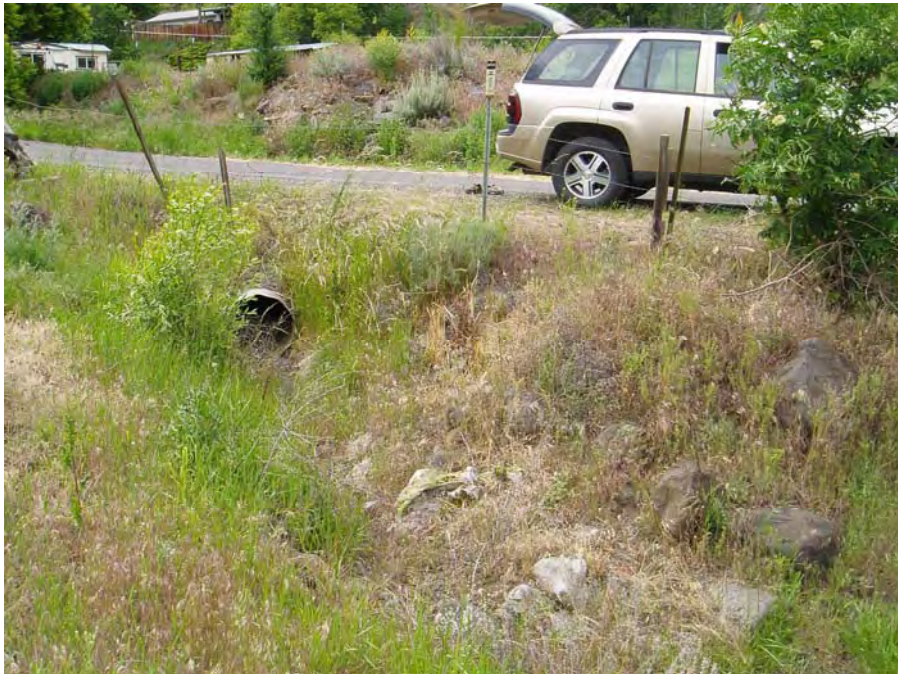
Photograph 2. Close up of the old mouth of Papoose Creek downstream of the culvert. This channel is now blocked by the road and the creek has been moved upstream of the culvert. Photo by D. Weigel, Reclamation.
