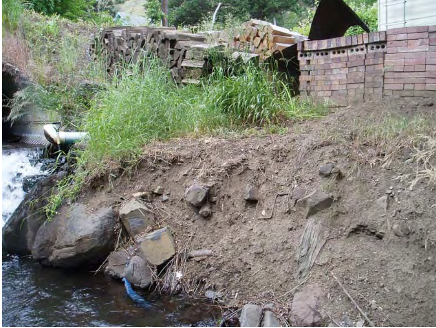
Photograph No. 3. Squaw Creek downstream of culvert. Landowner's property backs up to Squaw Creek. Photo by D. Weigel, Reclamation
