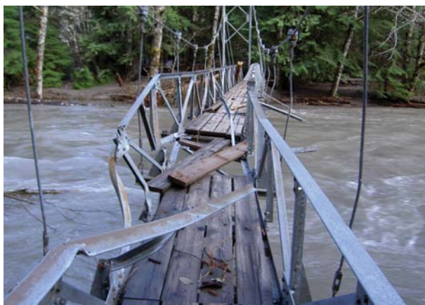
Suspension bridge across the Ohanapecosh River to the Grove of the Patriarchs
