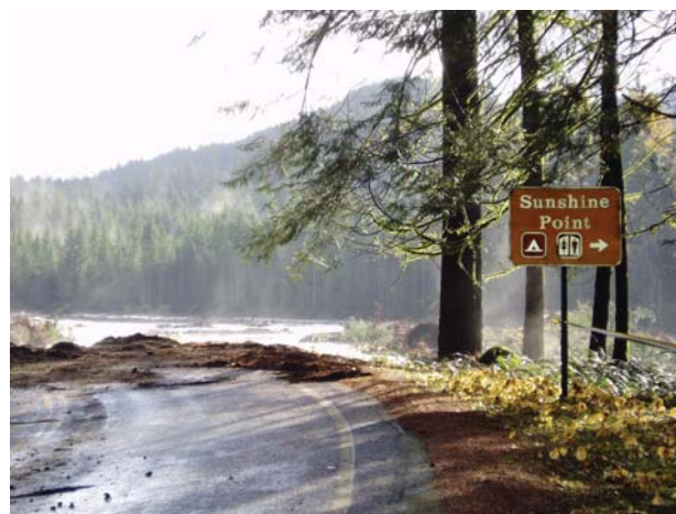
The Nisqually Road was washed out along with the former Sunshine Point Campground
