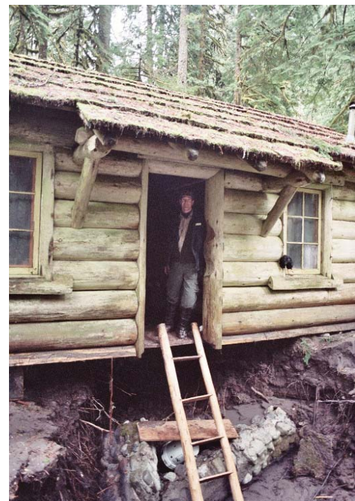
A channel of the Carbon River carried away the ground beneath the historic Ipsut Creek Cabin.
