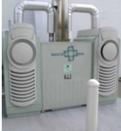
Figure 2: Capstone Microturbine with an Attached CHP Unit
