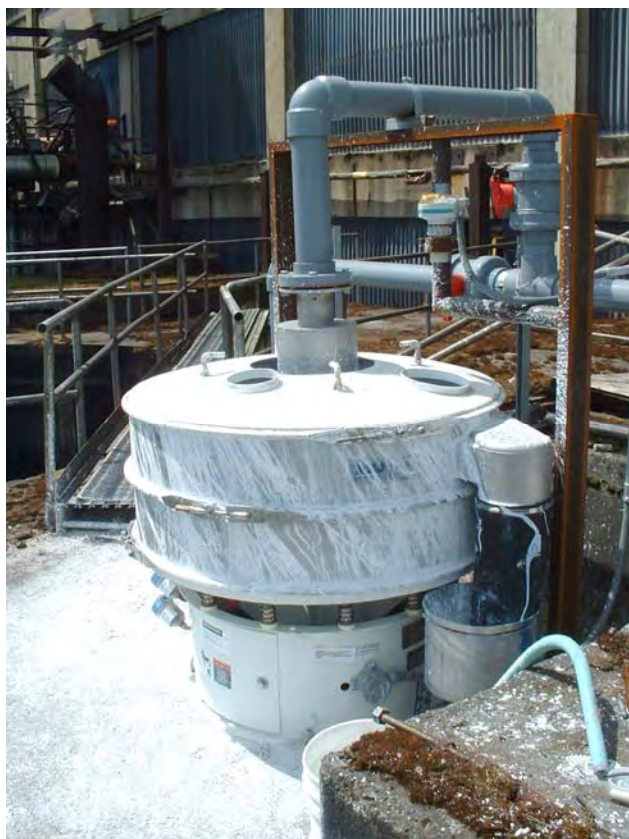
Figure I-3.15-5. Vibrating screen for product to remove reactor scale.
