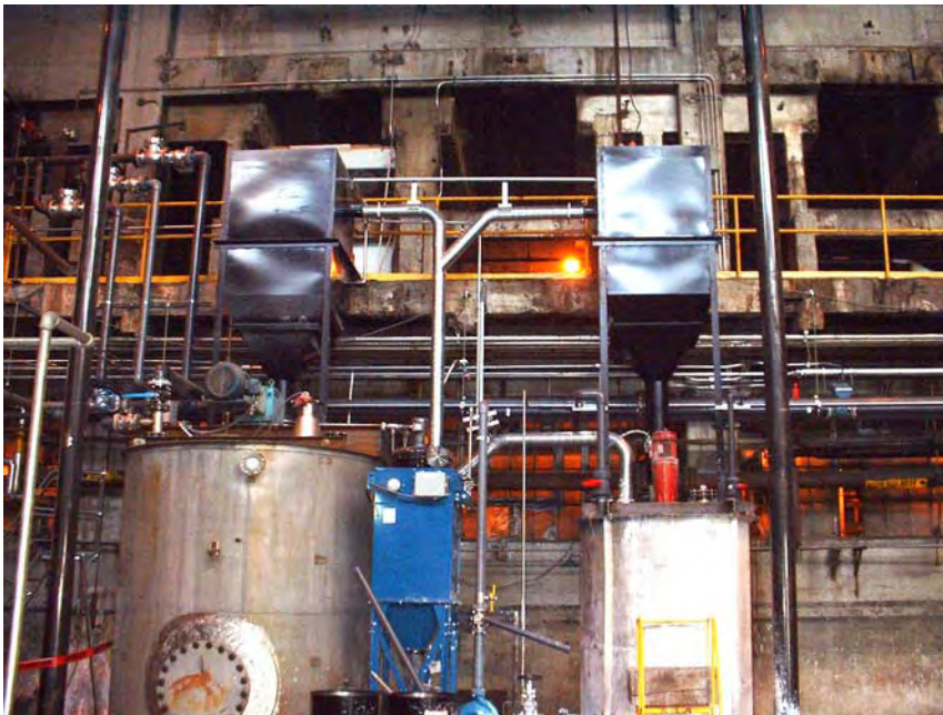
Figure I-3.15-4. DE mix tank and lime slaker with associated hoppers. Also pictured is the dust collection system for safe handling of lime and silica.
