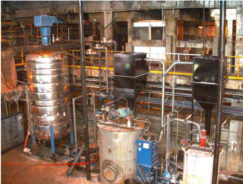
Figure I-3.15-7. Reactor, lime slaker, DE mix tank and all associated pumps, piping, hoppers and crane structure.
