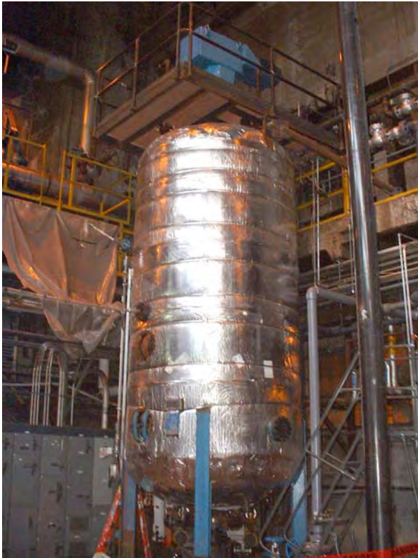
Figure I-3.15-1. Reactor for the prototype plant.
