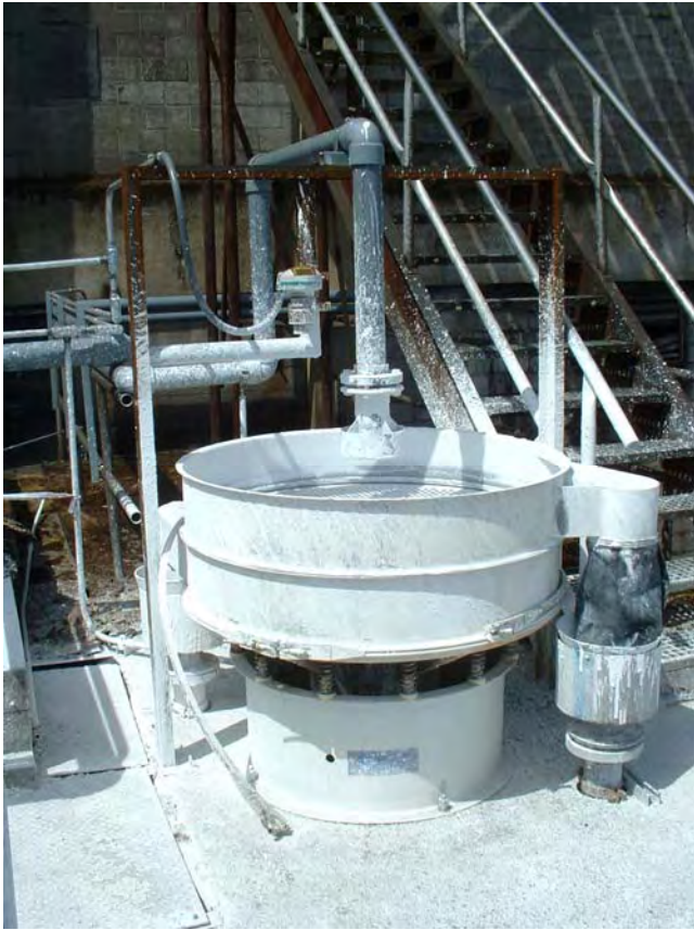
Figure I-3.15-3. Vibrating screen for lime preparation.
