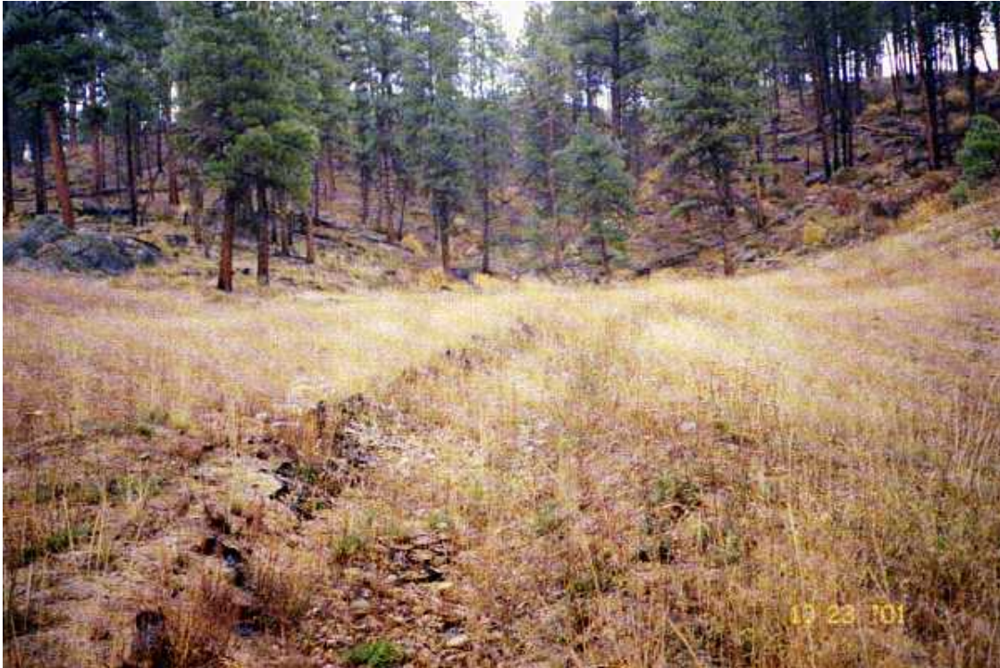
Photo 3. View upslope of GEOWEB cellular confinement system, filled with rock, in the collection ditch
