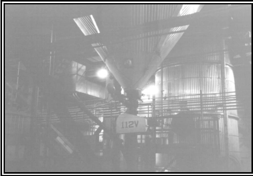
4.3b: Pyrolyzer Cyclone Fines Discharge.
