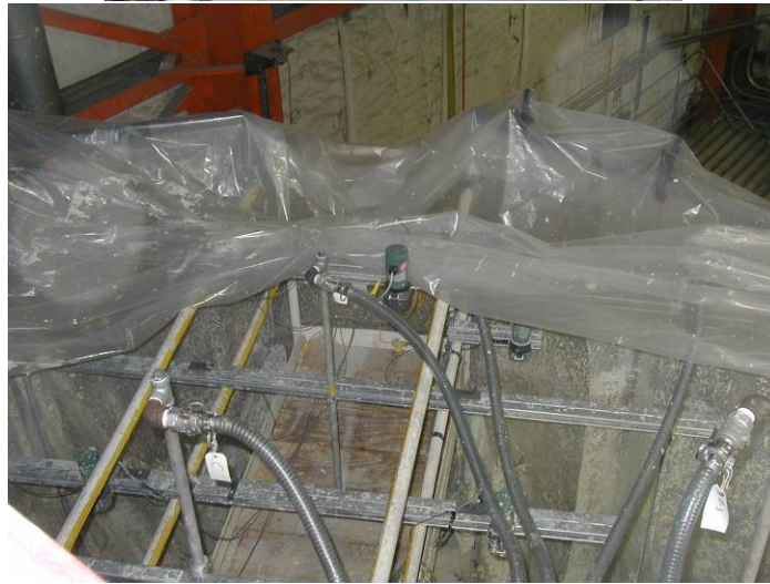
Figure 5.5. View of the Tank Top Configuration Showing the Walkway, Plastic Sheetting, and Several Sparge Tubes
