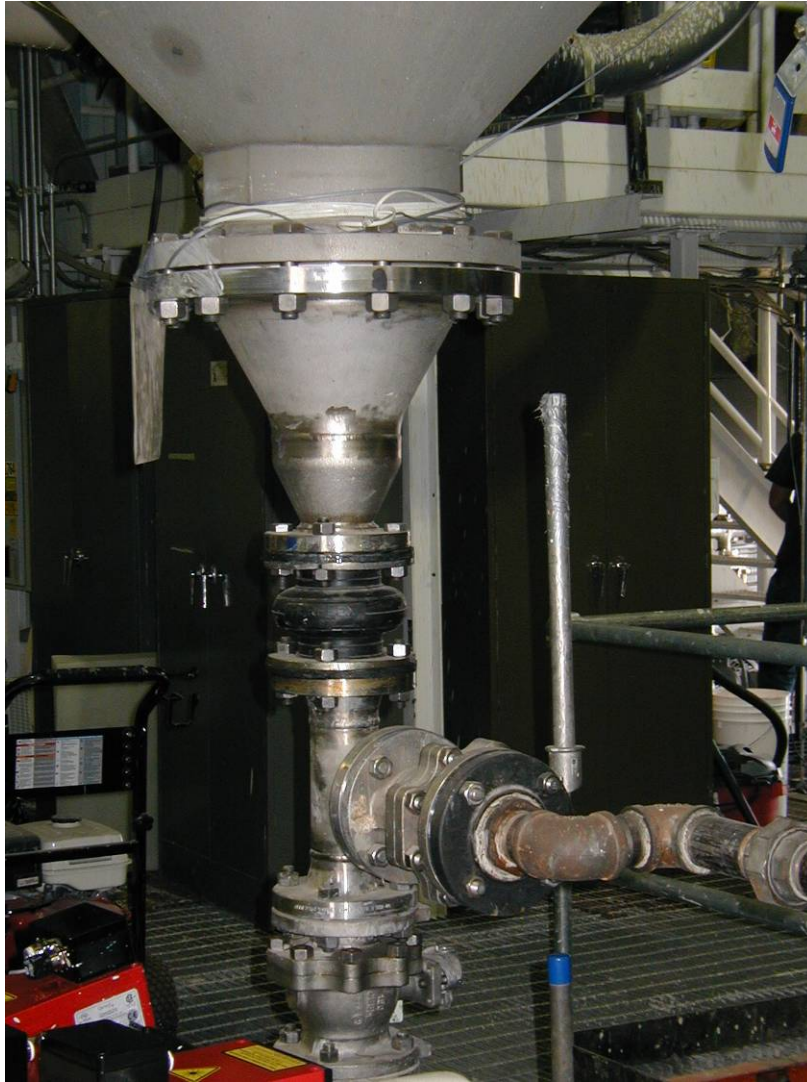
Figure 5.2. View of the CBT Tank Bottom Showing the Simulant Fill and Pump Out Line
