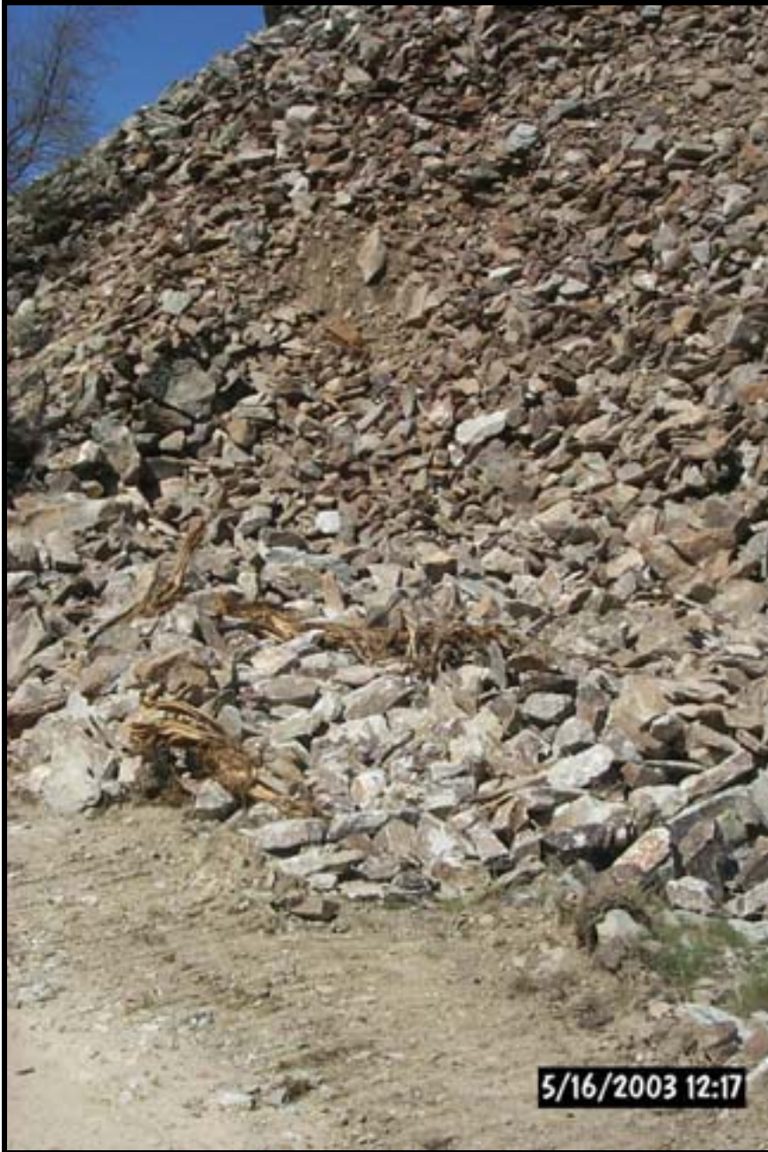
Photo 4. Areas of previous rock removal within the subject site. View to northwest.
