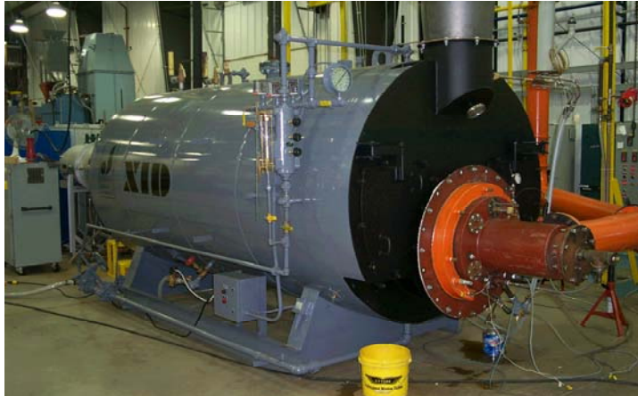
An Ohio Special boiler installed at GTI's Lab running at 250 BHP.
