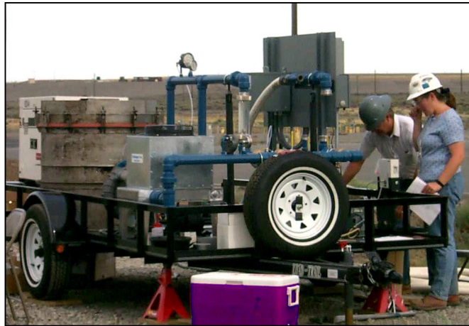
Subsurface CO 2 Sampling System
