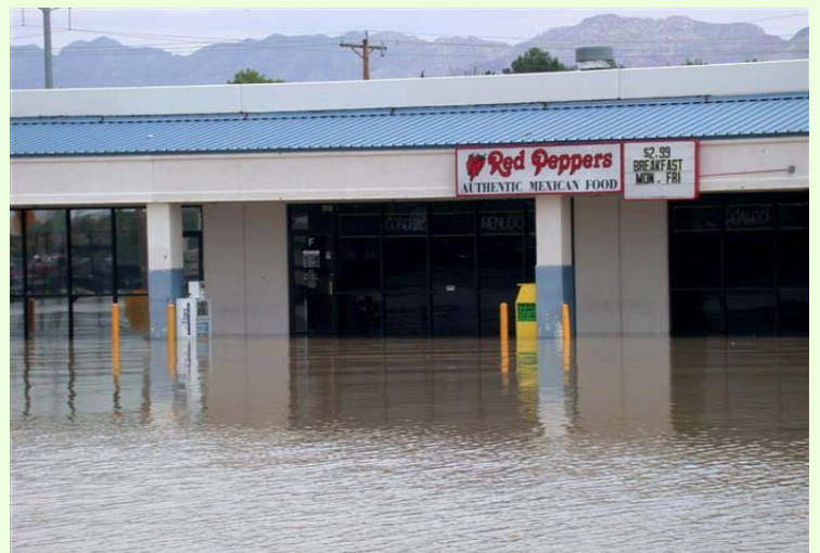
Strip mall flooding on Donaphan Street in west El Paso. (Photographed by Joe Rogash NWS)
