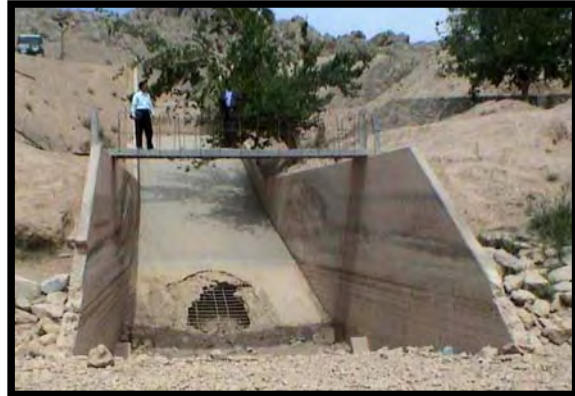
The damaged chute before repairs
