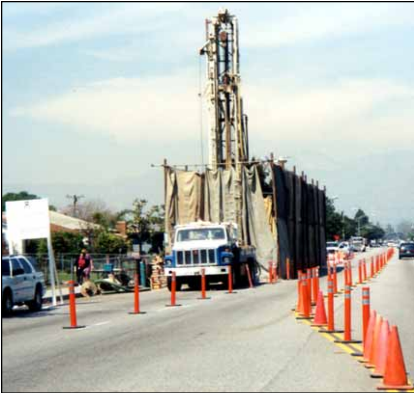
Figure 2: Typical Well Installation Site
