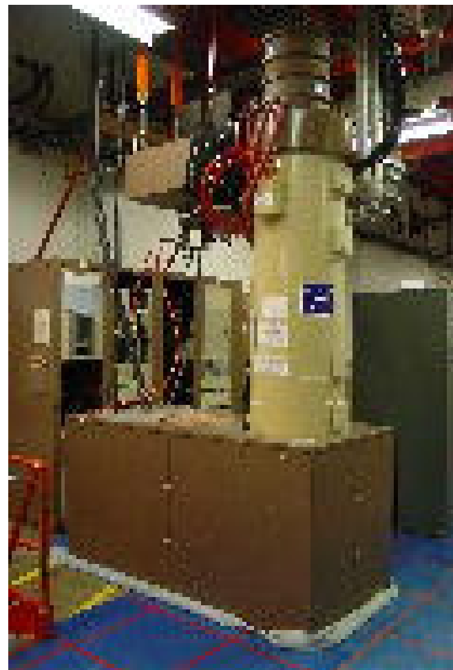
805 MHz 12 MW Klystron System
