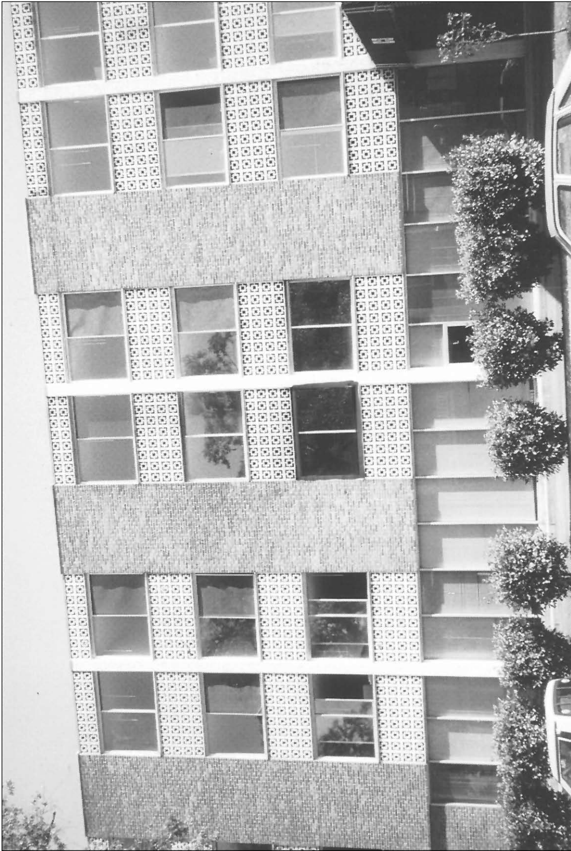
3. South end of building, indicating second floor window where fire originated.
