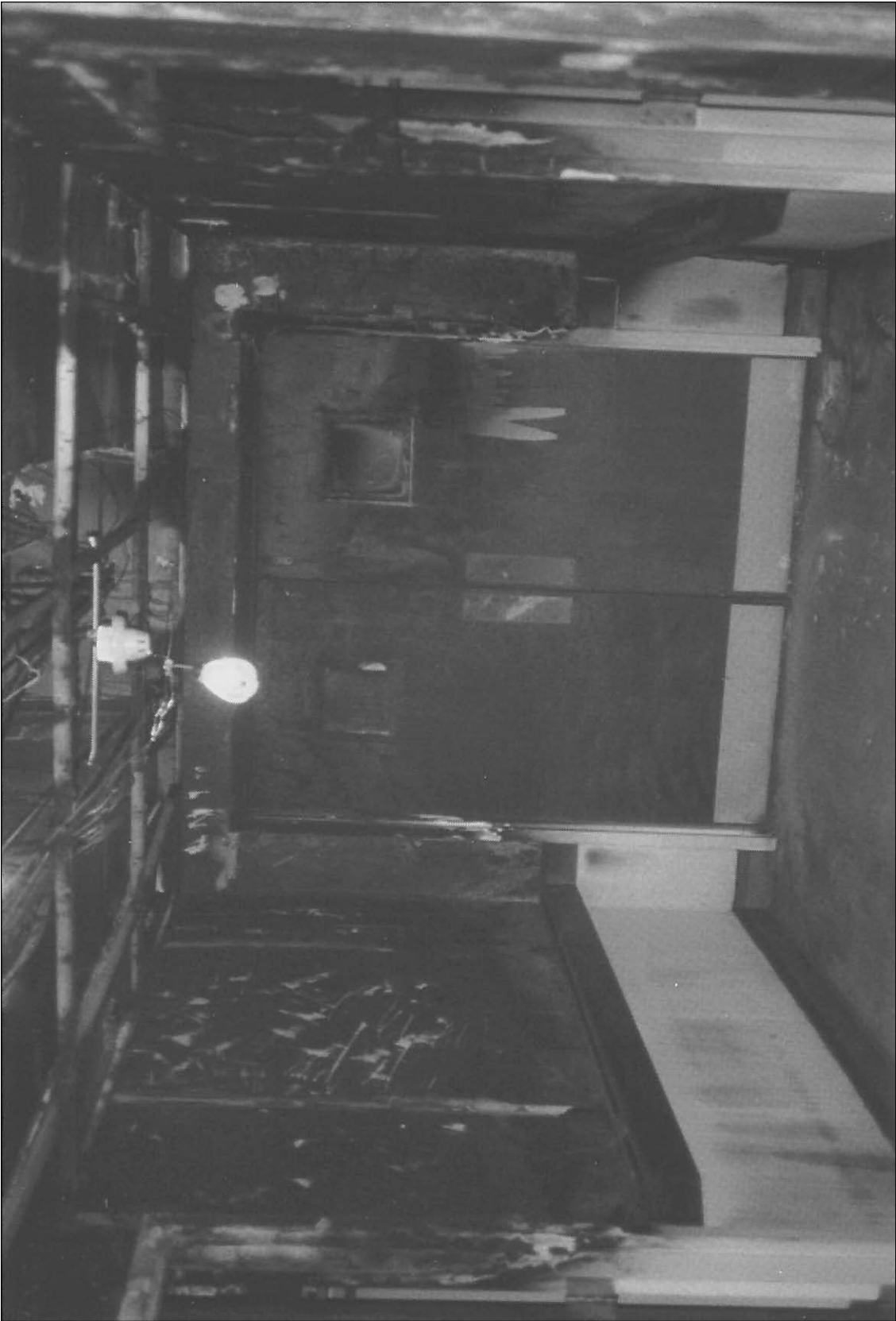
18. Fire damage to smoke barrier doors and to ceiling from room of origin on right.
