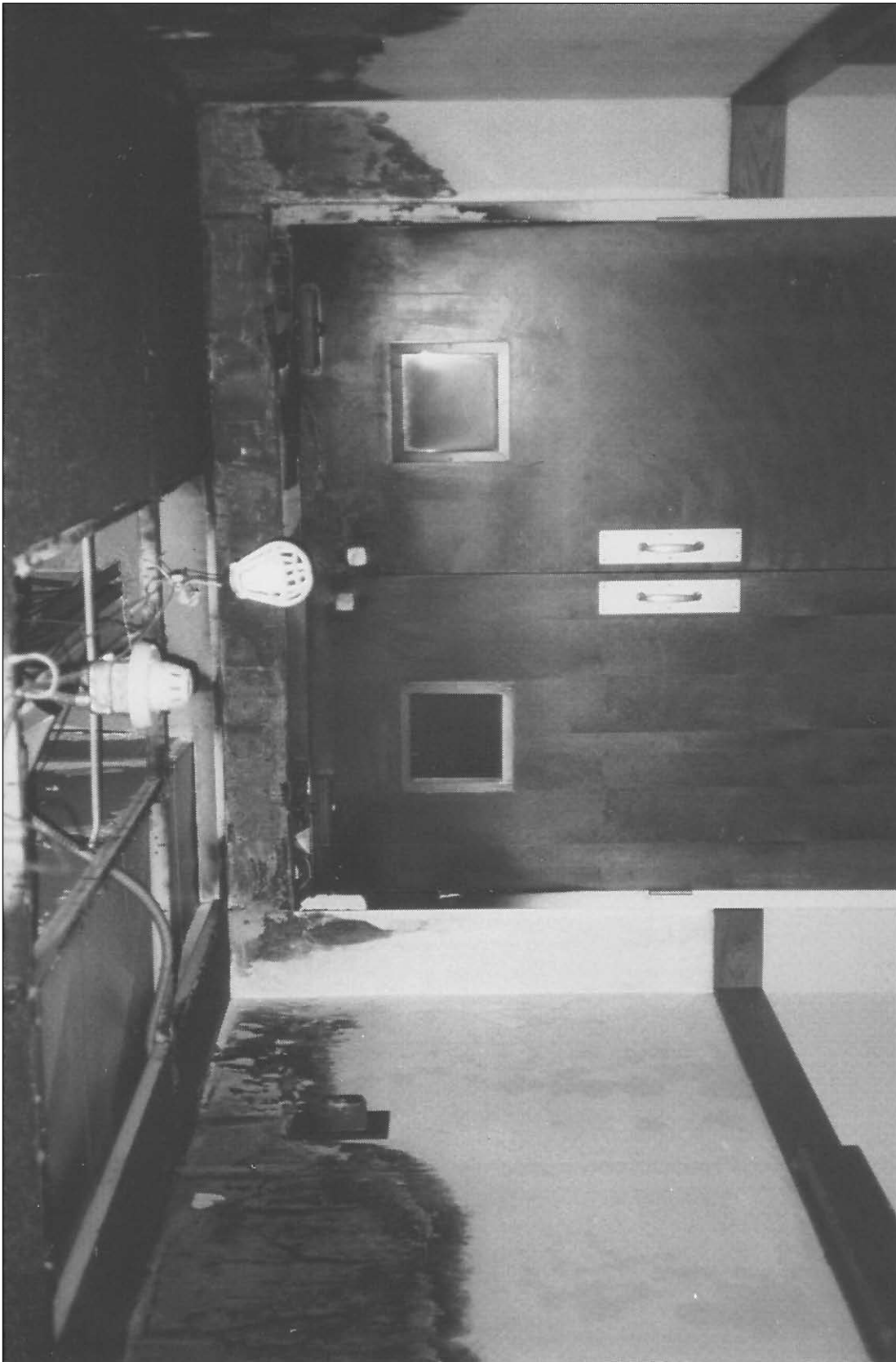
19. Fire and heat damage to ceiling and walls on opposite side of smoke barrier doors.
