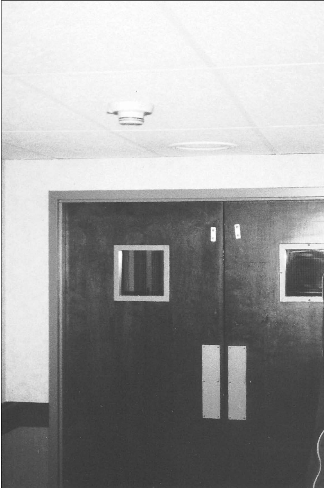
17. Smoke detector and smoke barrier located on second, third, and fourth floors.
