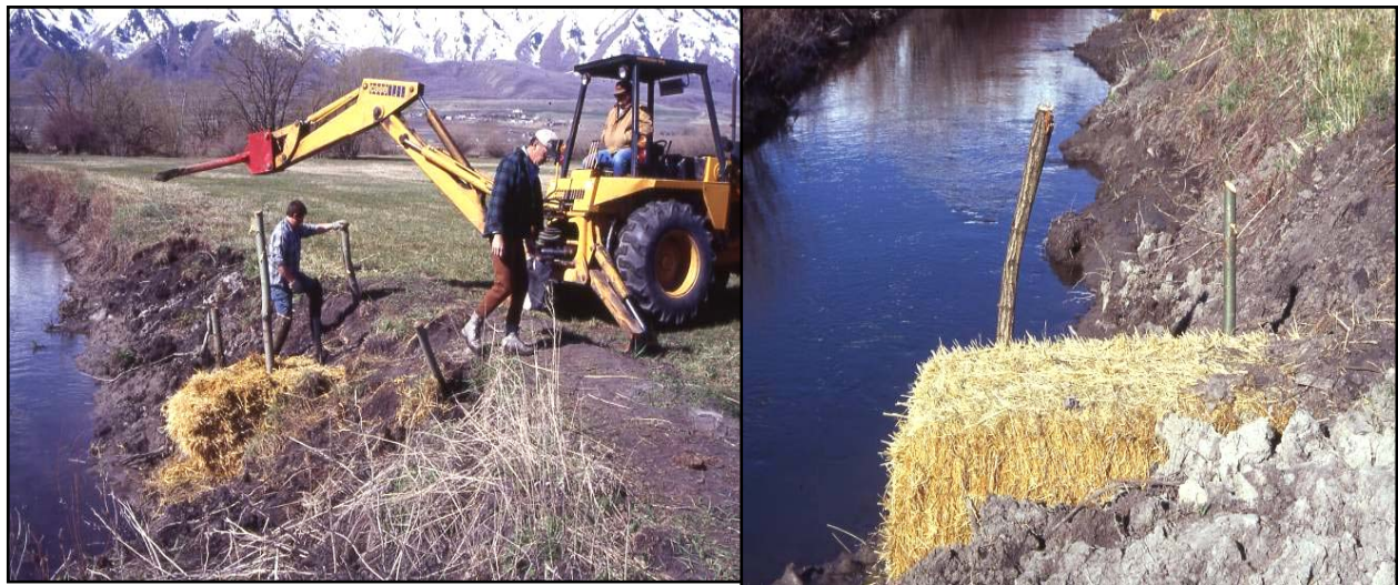
An example of an alternate use of The Stinger is pinning a hay bale to the bank so high stream flows will have a harder time removing them from the streambank
