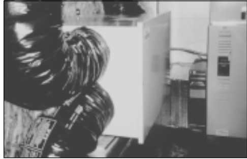
Figure 46. Heat recovery ventilation system.
