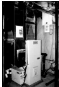
Figure 42. Interior geothermal equipment.
