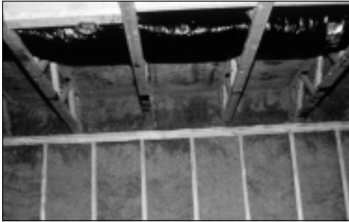
Figure 35. Ductwork in unconditioned space should be well-insulated.
