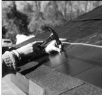
Figure 53. Workers install a photovoltaic shingle roofing product. The product installs just like asphalt shingles.
