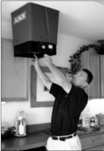
Figure 10. Duct leakage testing is less common than blower door testing but can also be used to demonstrate a home's energy efficiency. Tests can be performed on new houses before drywall installation at a cost of about $175 to $400.
