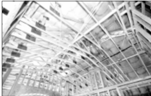
Figure 36. Insulation is attached to the rafters in this Las Vegas-area house featuring an unvented roof design.
