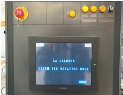
PLC controls Interlocks and Drum and Doors opening Fig. Q
