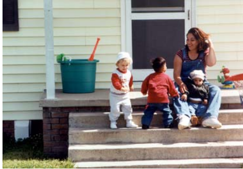
The small white box left of the porch is the only outdoor evidence of the new GHP system that provides heating, cooling, and hot water in this military family residence.
