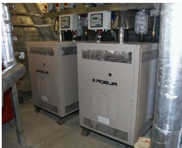
Figure 3: Absorption heat pump units.
