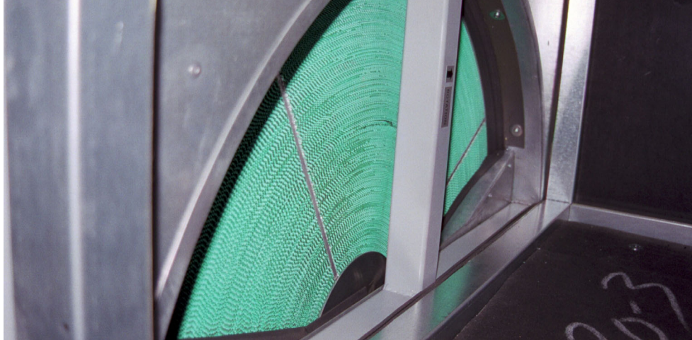
Fig. 2. The active desiccant wheel installed as part of the hybrid system at Berry College.
