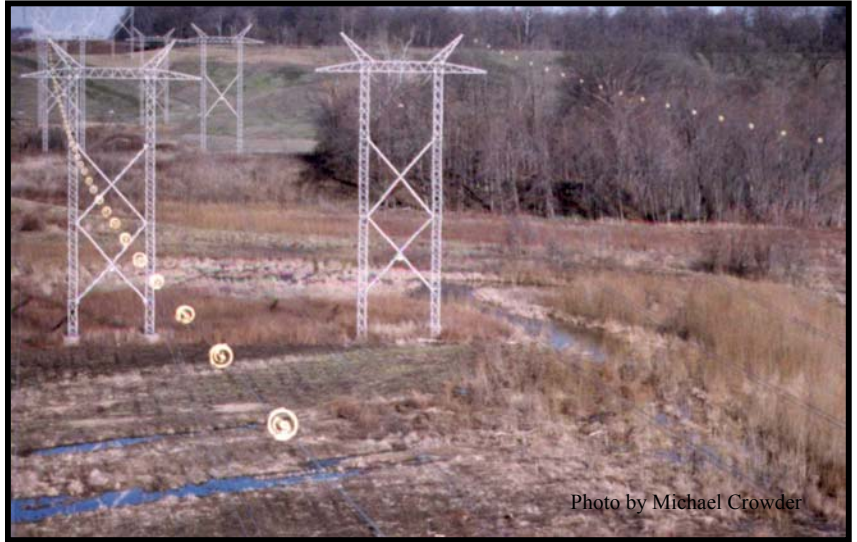
Figure 4-11 Swan Flight Diverters Installed at a 20-foot Interval in Indiana
