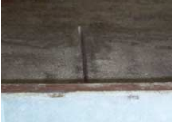
Figure 11. Photograph of crack sawn into the asphalt. The crack is 6 mm wide.
