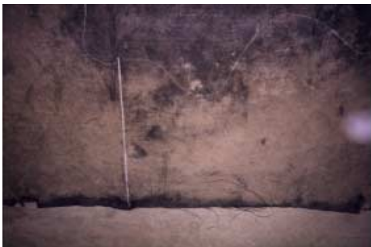
Figure 13. Photograph of the top of the geotextile separator removed from the control section. Staining with soil fines appears to indicate where significant amounts of water flowed through. The location of the crack in the asphalt is highlighted with the chalk line. The black edge suggests that no water migrated across the edges of the separator.
