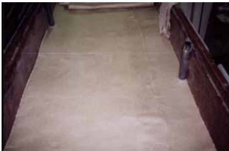
Figure 14. Separator layer of GCBD after placement on the subgrade. Note overlap of the geotextile towards the right side of the box.
