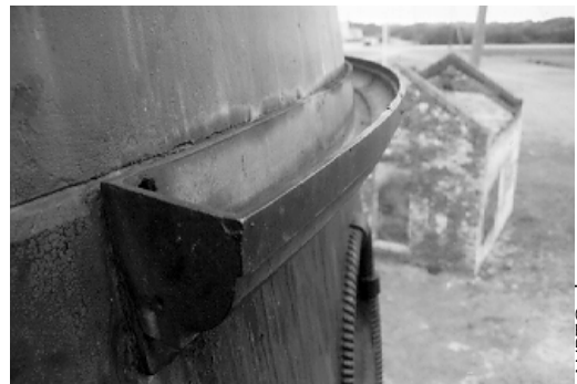
Figures 23 and 24. Two types of gutters found on iron lighthouses; the gutters must be in proper working order and checked regularly during the mothballing period.
