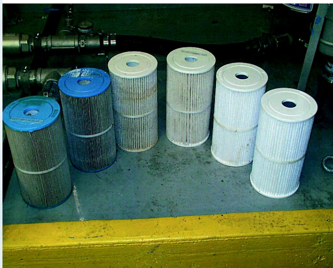
Figure 6-14. Dirty and clean cartridge filters.
