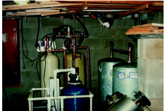
Figure 7-2. AOP POE unit installed in a cellar.
