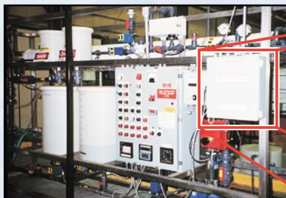
Ultrafiltration System (After)
