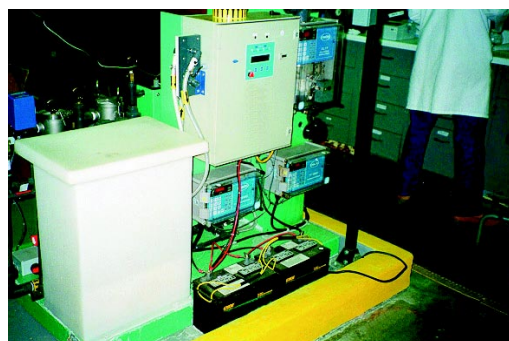
Figure 6-24. On-Site Chlorine Generator #2.
