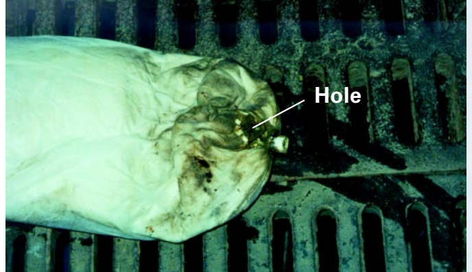
Figure 6-6. Bag filter showing fabric rupture.
