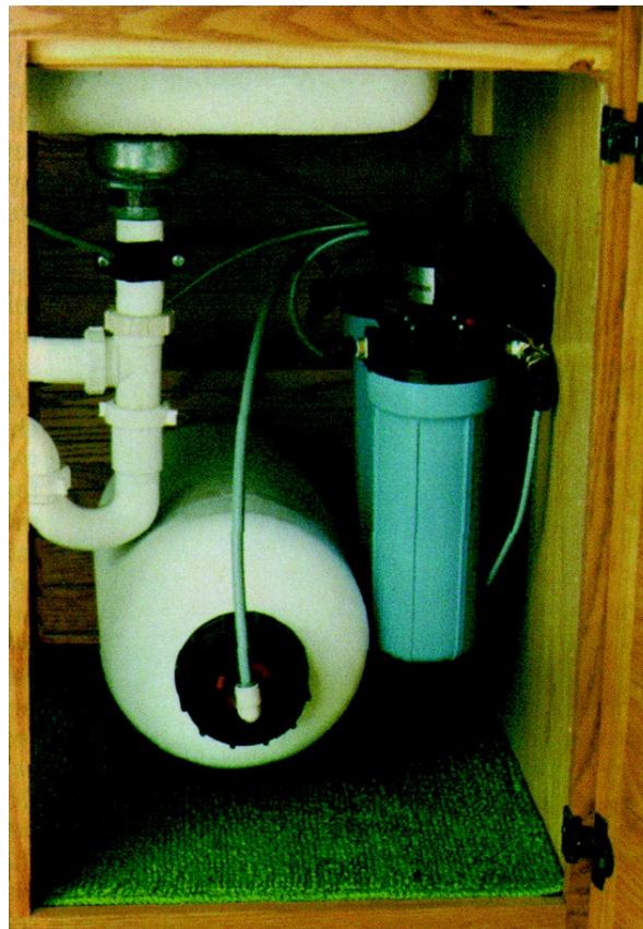
Figure 7-1. Typical RO Unit under a kitchen sink.
