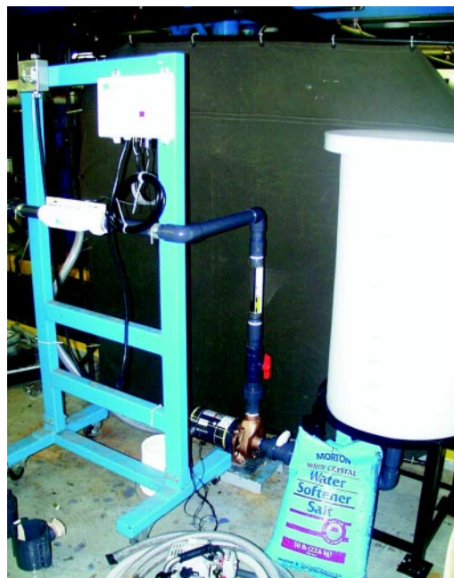
Figure 6-23. On-Site Chlorine Generator #1.
