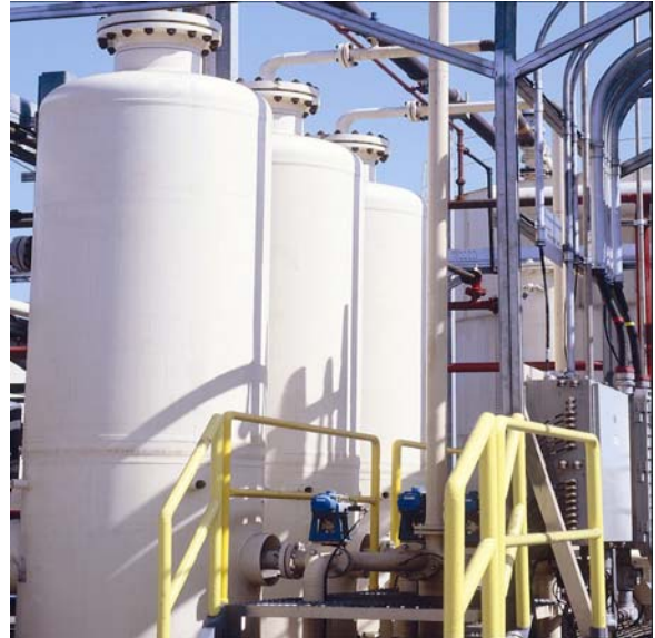
Figure 4. Tidelands Oil Facility. Engelhard's Molecular Gate molecular sieve is contained in a series of pressure vessels. The separation and purification process occurs within these pressure vessels.
