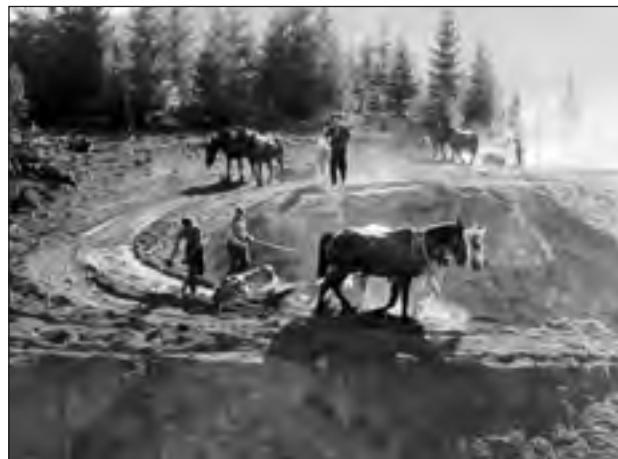
CCC Company 944 from Camp Hemlock and a horse team working on a new road.
