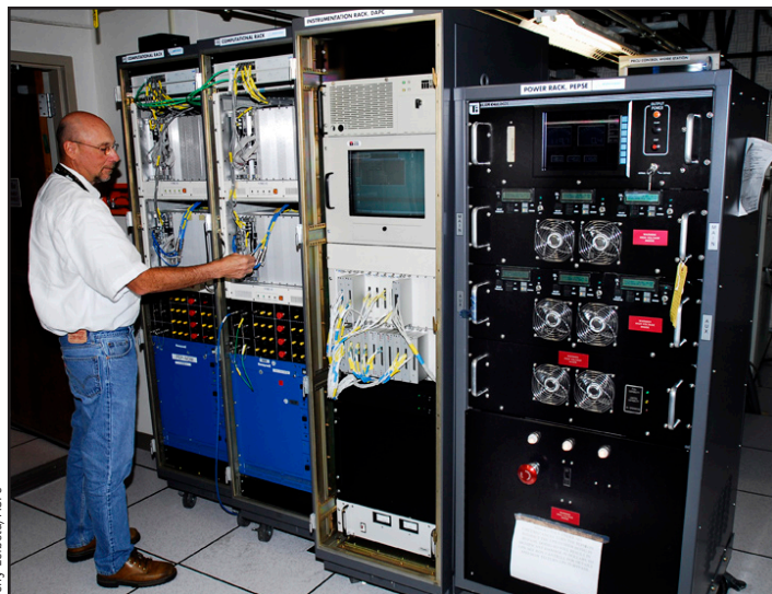
Bill Telesco, payload rack officer, checks cables connecting to the Payload Rack Checkout Unit from the EXPRESS Rack.
