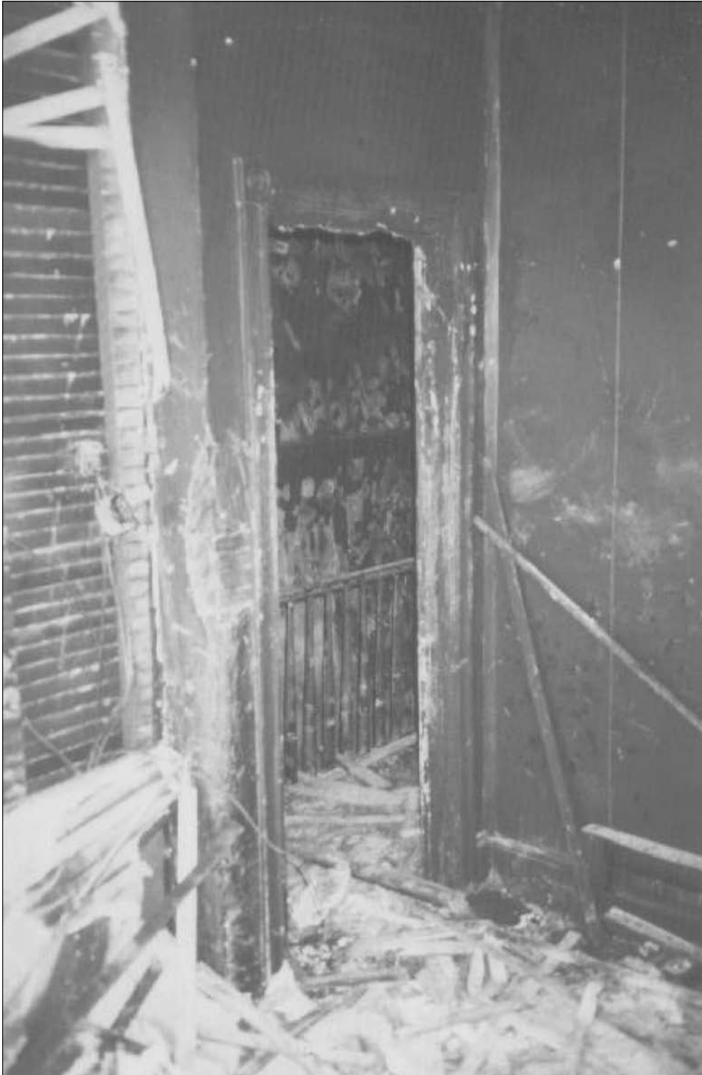
Entrance to second floor rear bedroom looking towards hallway. The door trim detail remains intact and heavy smoke residues stain the interior walls.
