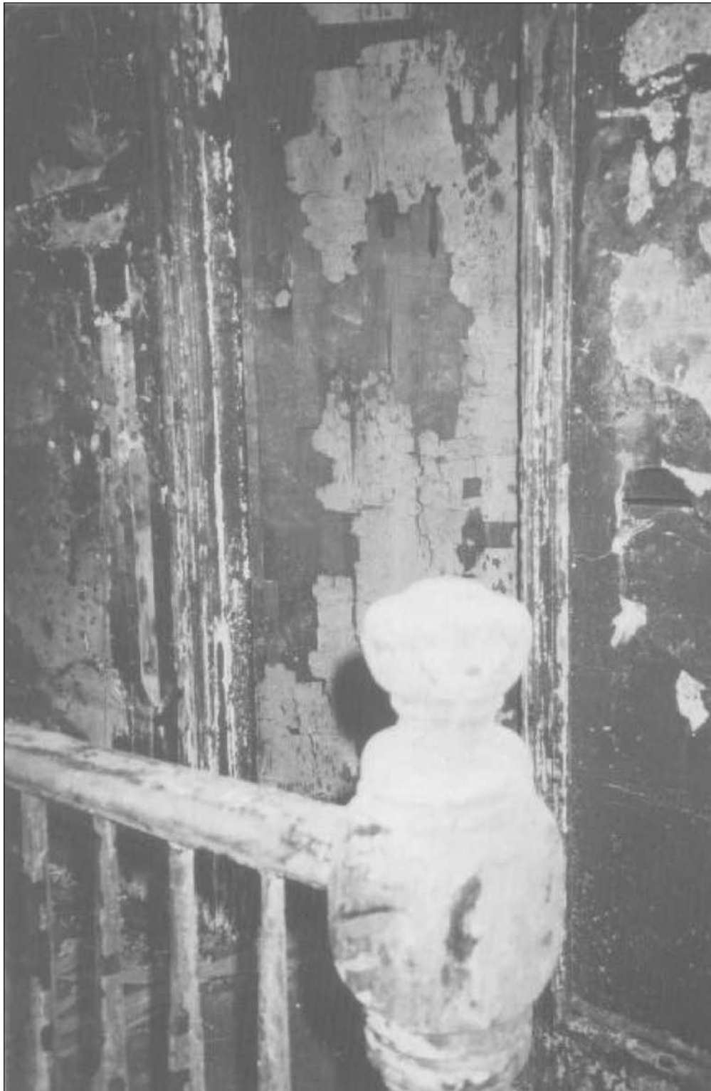
Rear doorway to second floor center bedroom. The homemade door is partially delaminated, explaining the irregular burn pattern.
