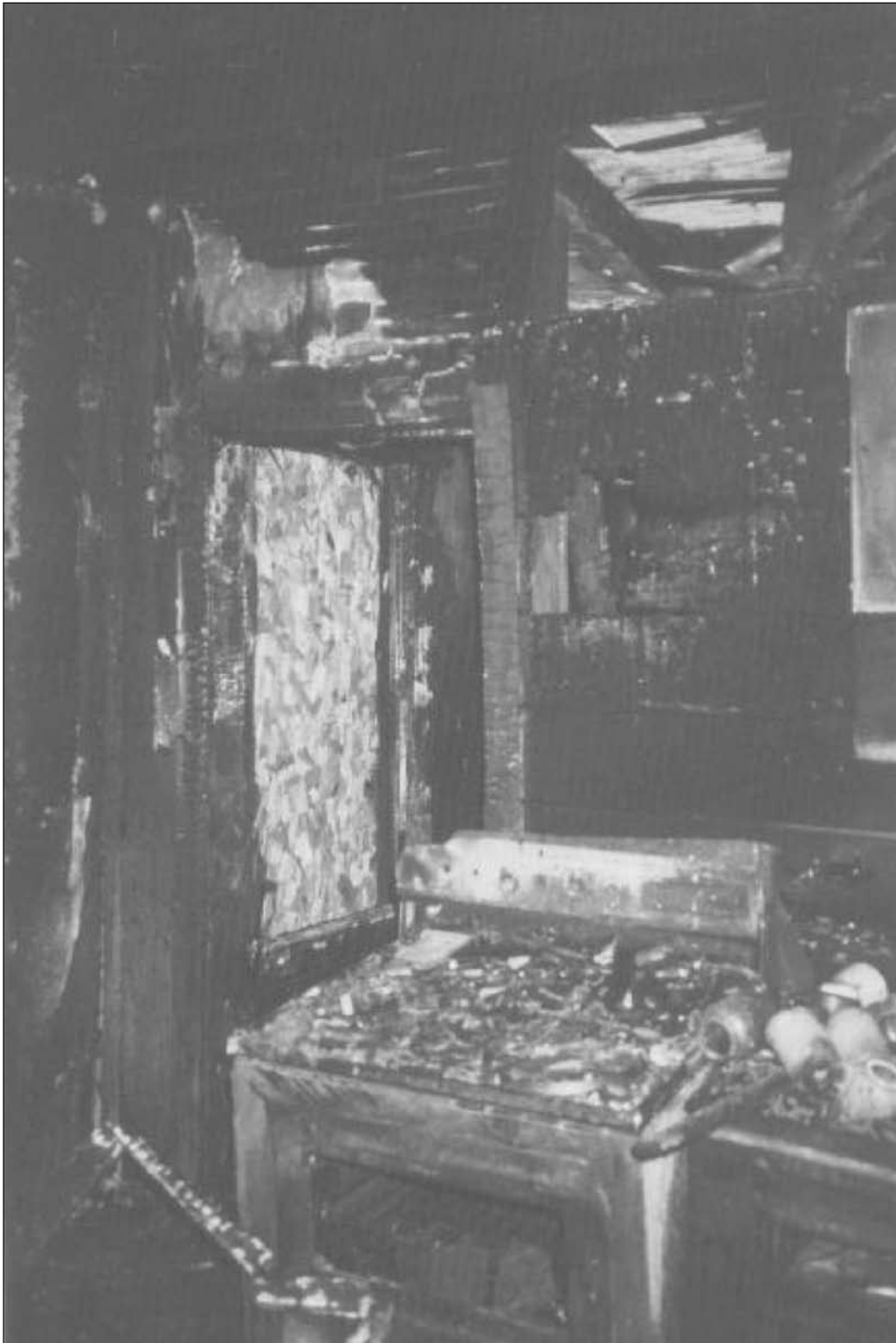
Fire damage in the kitchen area looking towards the rear hallway leading to the rear bedroom where the fire started.
