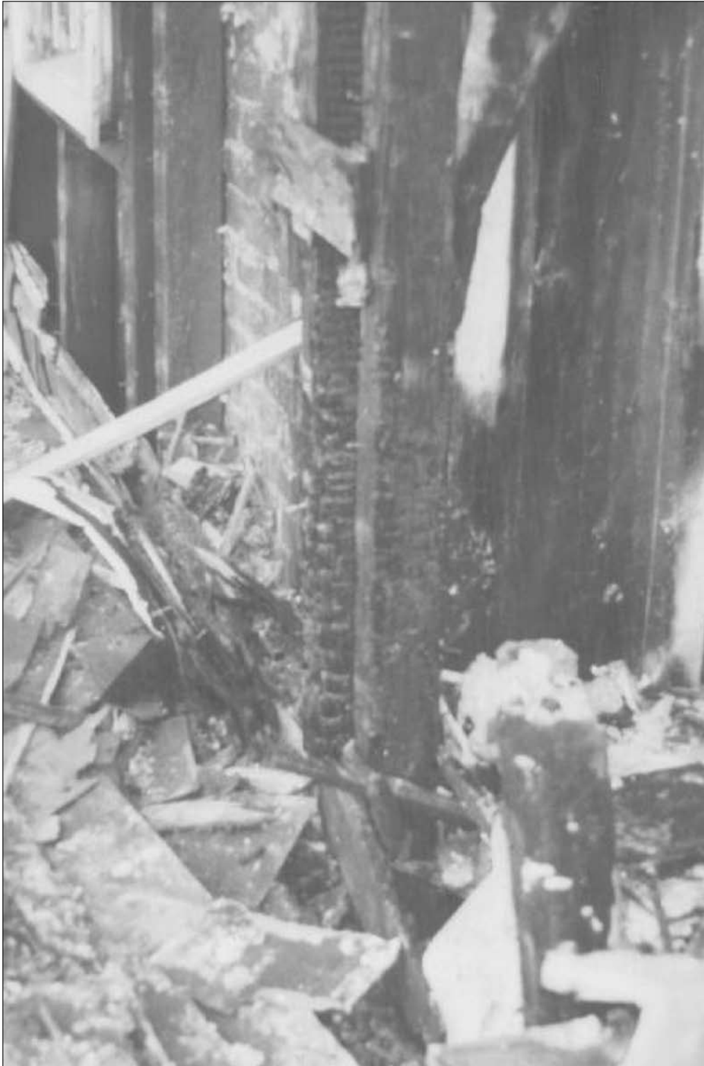
Charred stud in exterior wall of second floor rear bedroom. No firestopping was provided between the first and second floors. This is typical of balloon frame construction.
