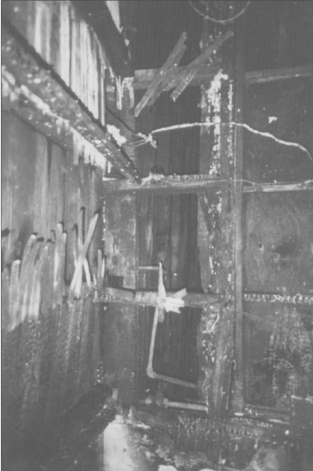
Wall and ceiling area above point of origin. Voids in the wall construction where the ceiling joists were attached permitted the fire spread horizontally into the kitchen and vertically into the rear exterior wall of the bedroom above.
