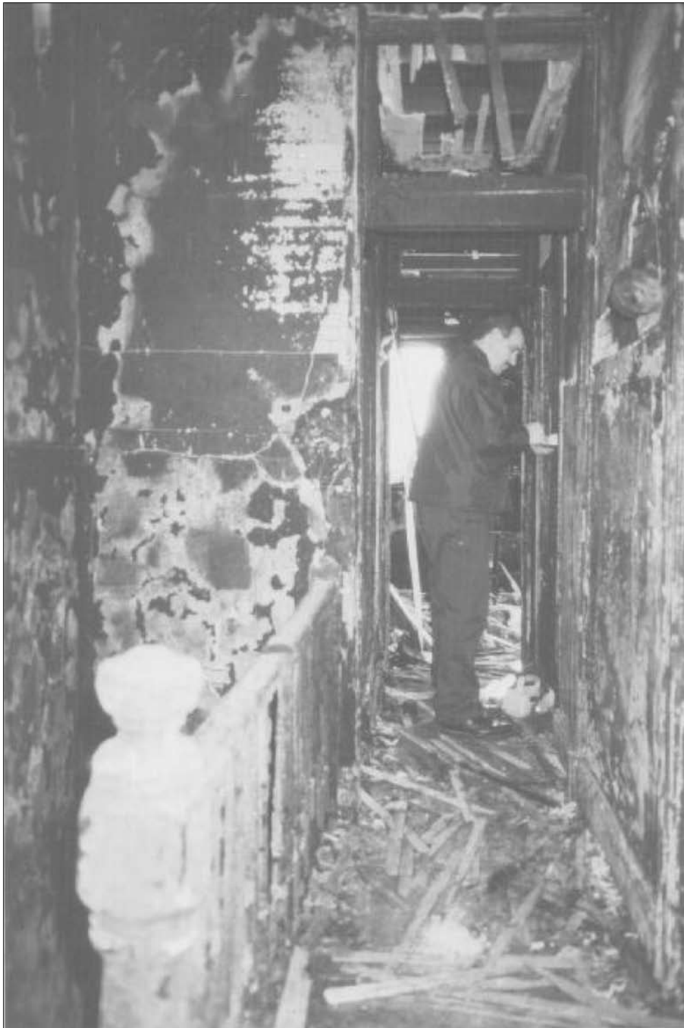
Second floor hallway looking toward front (master) bedroom. The burn pattern on the wall above the stairway opening is evidence of flame rollover from the intense fire in the dining room, kitchen, rear hallway, and bedroom below.
