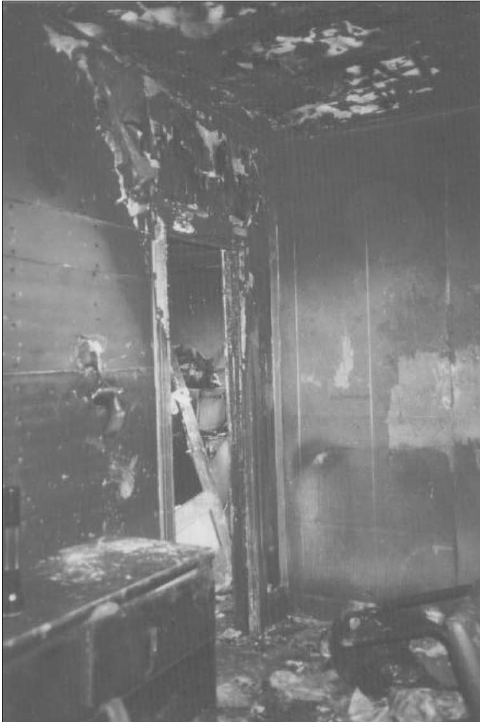
Thermal damage to wall and ceiling at top of front door opening to second floor center bedroom. This doorway was closed during the fire. However, convected heat and smoke from the fire below (see previous photograph) infiltrated the doorway through air gap at the top of the door.
