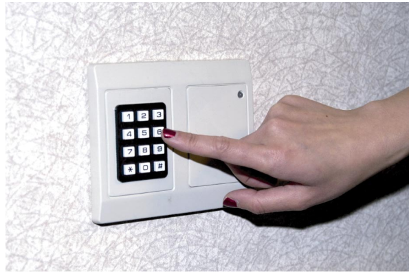
Keypad entry system.
