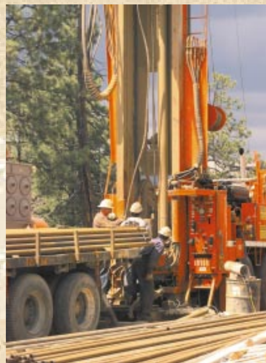
Drilling activities for well R-25 were completed in early 1999. This well is located in Technical Area 16 (TA-16), where operations include high-explosives research, development, testing, and manufacturing. Discharges from past manufacturing activities at TA-16 appear to be the source of high-explosive constituents discovered in the groundwater sampled from this well.
