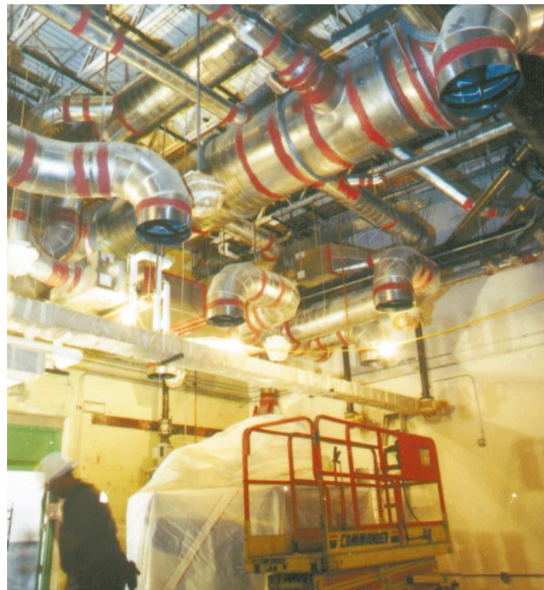
The complex, state-of-the-art ventilation system at the new Beryllium Technology Facility is just one part of the Laboratory's Beryllium Disease Protection Program.
